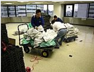
pack the cable trench steel caps
