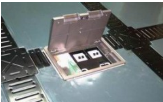
To accommodate large size floor box - Cut at side of the panel (count in the Cable Trench width) and installed at the trench.
